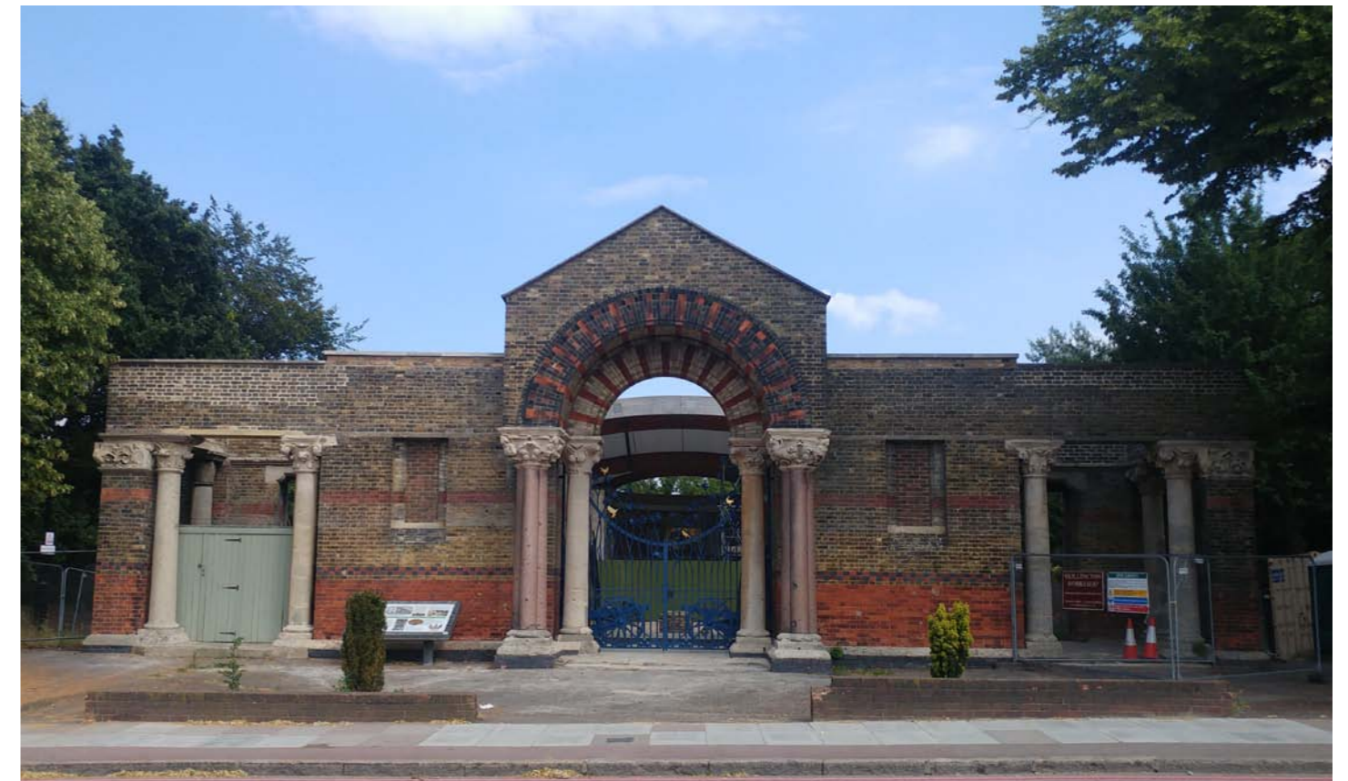
Below: Phase 2 Works; Brick and Stone cleaning to the main entrance facing Grand Depot Road and the Parade Ground.
